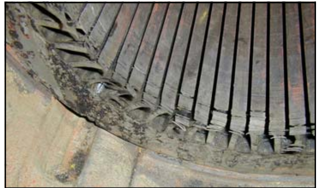
An example of end laminations damaged during coil removal.
