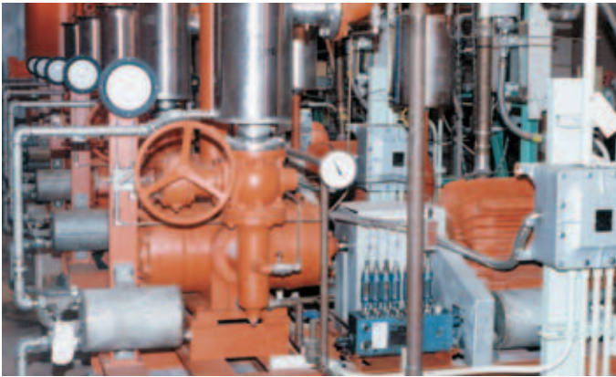
Five (5) model 8DB Ro-Flo® compressors, each unit compressing 220 acfm of municipal digester gas from 14.3 psia to 55 psig at the Cedar Creek WWTP in Nassau County, NY. The compressors are direct driven by 60-hp electric motors at 1182 rpm.
