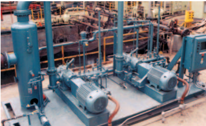
Two (2) model 10GB Ro-Flo® compressors recovering 500 Mscfd of hydrocarbon vapors from 0 psig to 46 psig for Thums-Long Beach, CA offshore unloading station. The compressors are direct driven by 60-hp electric motors at 865 rpm.
