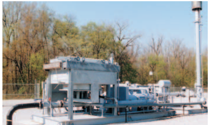
One (1) model 19L Ro-Flo® compressor compressing 1979 acfm of landfill gas from 0.5 psig to 25 psig for LFG Specialities at National Serv-All Landfill in Fort Wayne, IN.
