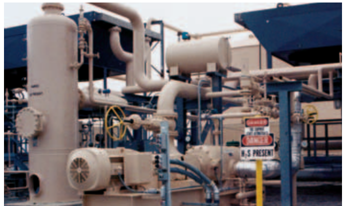
Four (4) model 19L Ro-Flo® compressors, each compressing 2300 Mscfd of wet CO 2 and H 2 S from a tank battery at Aera Energy LLC (formerly Shell Oil Co.) in Kern Ridge, CA. The gas is being compressed from 12.0 psia to 43 psia using 250-hp electric motor with a variable-frequency drive.
