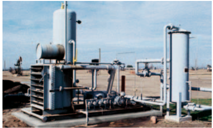
One (1) model 8DE Ro-Flo® vacuum compressor, boosting 340 Mscfd of wellhead gas from 10 psia to 45 psia for Exxon's Hershey Lease, Bakersfield, CA. A 50-hp electric motor drives the compressor at 1465 rpm through a V-belt drive.
